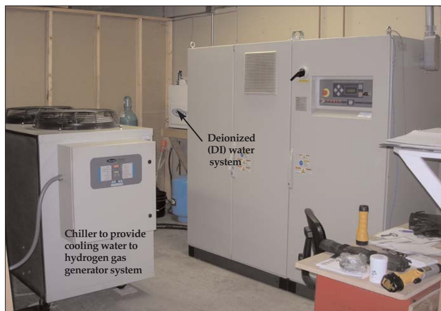
Chand Eisenmann Metallurgical's Hogen on-site hydrogen gas generator system installation.
